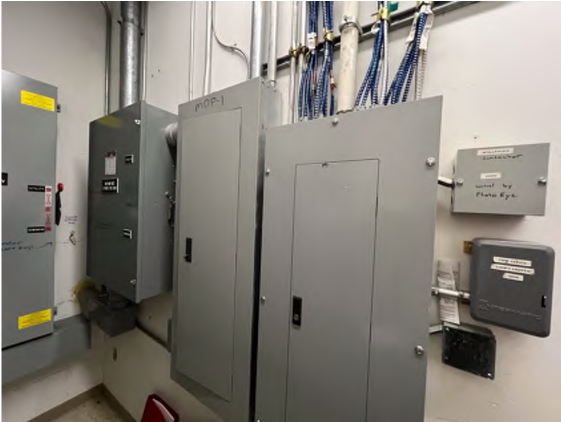
Figure 1. 400A service side at electrical room.
