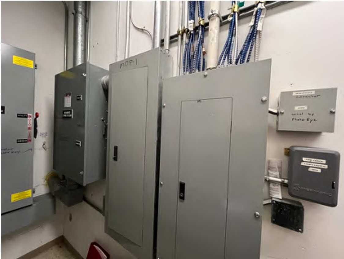
Figure 1. 400A service side at electrical room.
