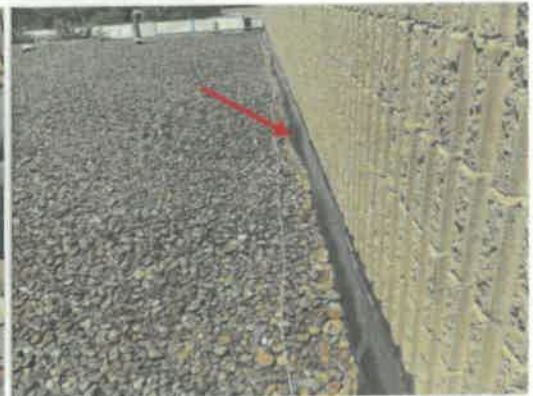
16. Membrane bridging was noted along several rising interior walls. This occurs due to membrane shrinkage and the lack of adequate termination of the membrane. The membrane should be cut, allowed to relax and stripped in.
