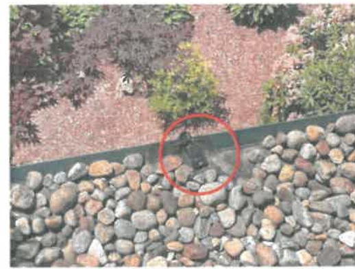
11. Open flashing noted at the perimeter edge. Provide new EPDM patch in accordance with Carlisle guidelines.
