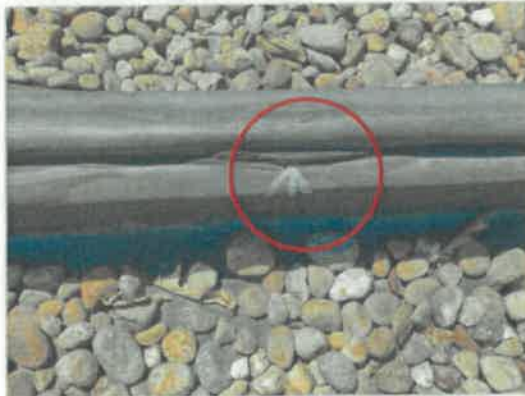
15. Open membrane seam on expansion joint. Provide EPDM patch in accordance with manufacturers guidelines.
