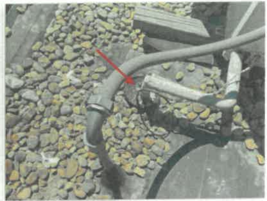
14. Deteriorating pitch pocket. Pitch pocket should be filled with an appropriate pourable sealant.
