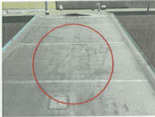
13. Soft insulation below roof membrane. These areas should be monitored to ensure that the area of soft insulation does not expand. It may be advisable to have an infrared scan completed to determine if the roof insulation in these areas is wet.
