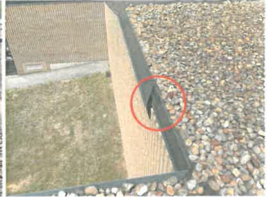
20. Loose edge metal flashing. This edge metal should be resecured.
