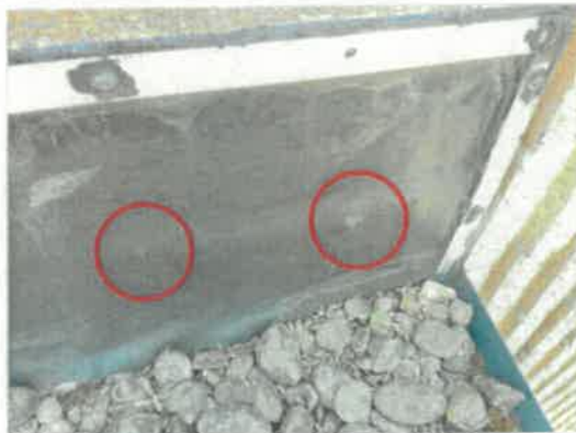
17. Tented fasteners were identified in several areas of the facility. Provide EPDM patches over these fasteners in accordance with Carlisle guidelines.
