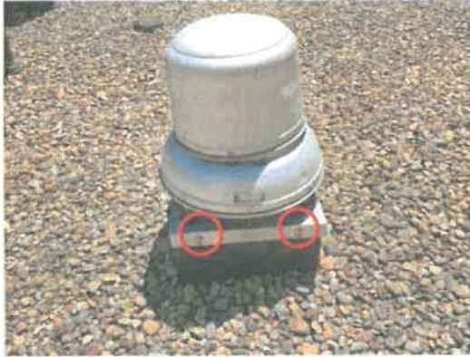
7. The majority of the roof top fans were noted to have missing or non-grommited fasteners. Grommited fasteners should be provided at each attachment point. Existing non-grommited fasteners should be caulked.
