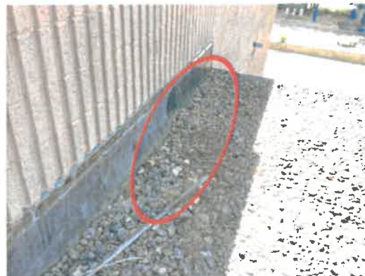
23. Organic growth should be removed during annual roof maintenance.
