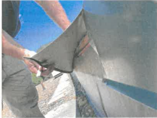
12. Metal edge fascia with no hook strip or dutch clips. This fascia should be secured to the plywood with minimum No. 8 grommited screws at 16 inches on center. These fasteners should be installed along the lower 1/3 of the flashing.
