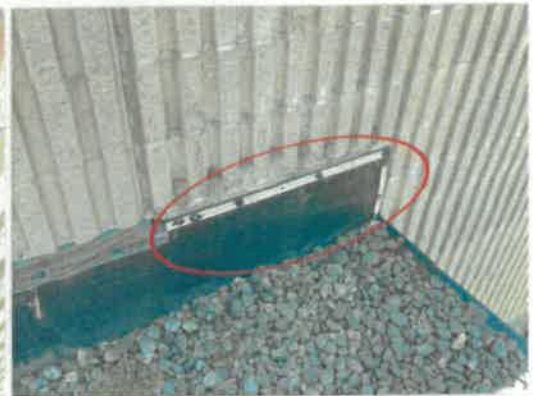
18. Missing through wall flashing cover. Provide caulking over this entire termination bar to provide a water tight condition.
