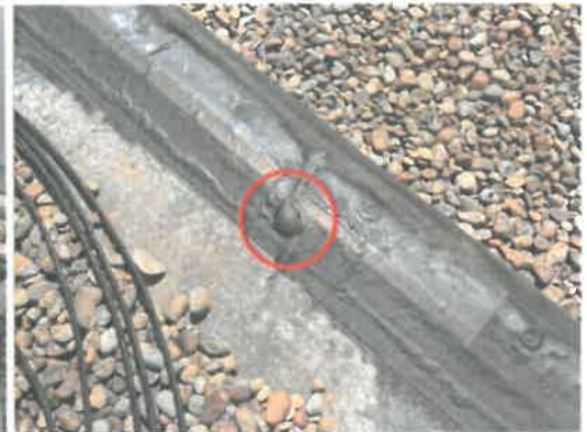
22. Blister on EPDM stripping at roof perimeter. Provide new EPDM patch in accordance with Carlisle guidelines.
