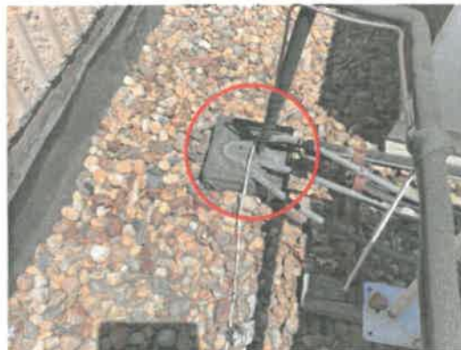
21. Pitch pocket with multiple cables. The pourable sealant has deteriorated, and Karnak has been applied. These materials are not compatible, and the pitch pocket should be reworked with an appropriate pourable sealant.
