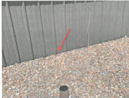
9. Low flashing height was noted in several areas. These areas should be monitored to ensure that these areas do not become prone to leaking. If no problems appear, these flashing heights should be addressed during new construction.
