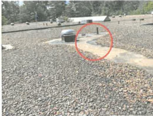
19. Evidence of roof ponding was identified in several roof areas. These areas should be monitored to ensure that the ponding does not worsen to the point that the roof insulation is damaged.
