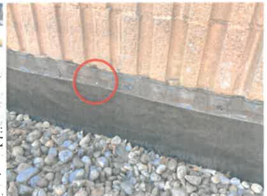
24. Uncaulked rivets were noted at the base of several rising walls. Provide caulking of these rivet in accordance with Carlisle guidelines.
