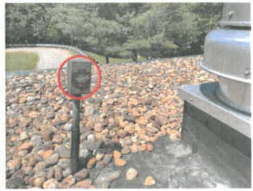
10. Open electrical boxes should be sealed per local code. An alternative would be to remove the electrical boxes and conduit and the roof should be repaired in accordance with Carlisle guidelines.
