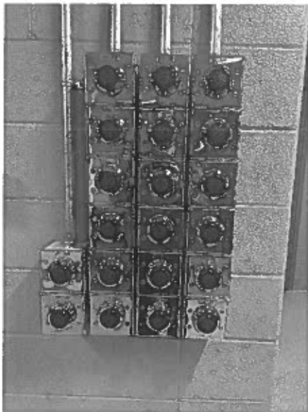
Toilet Flushing Control Station (Brockton PD)
